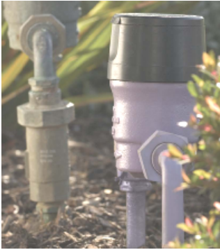
Figure 2: Recycled (Lilac) and Potable Water Meters
