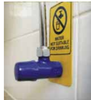
Figure 5: Toilet Tap and Labelling
