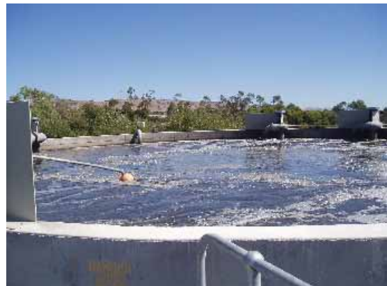
Willunga Wastewater Treatment Plant
